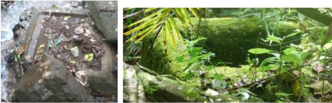
The two different collection chambers of the first catchment
