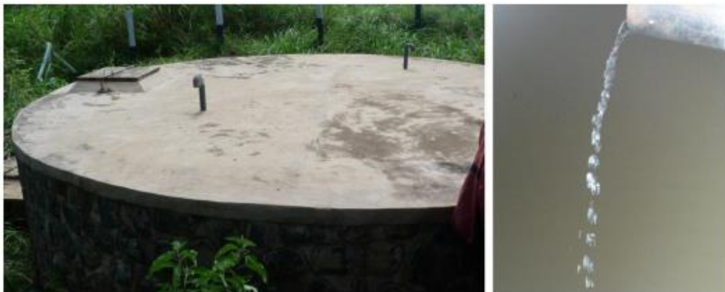
The distribution tank, which is supposed to supply the entire village with water, and its intake pipe
