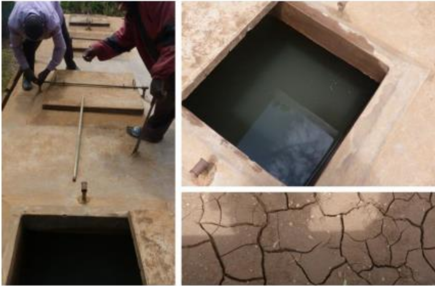
The treatment tank, shown during the rehabilitation work. In the upper right-hand corner, a photo of one of the individual chambers. Beneath that, an image of the removed mud from sedimentation chamber.
