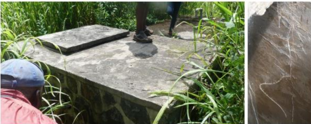
Unused storage tank and roots growing in the tank
